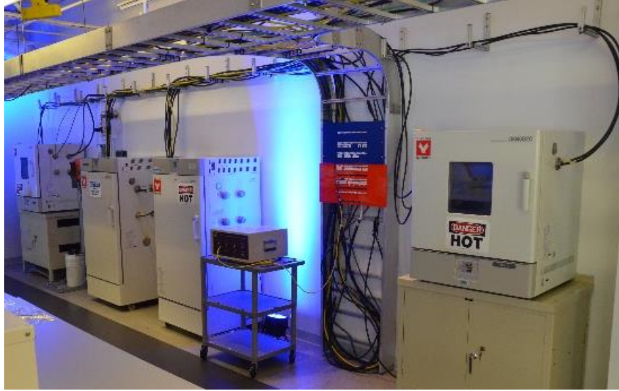
Figure 2. AMS Aging Ovens and Cable Raceways
