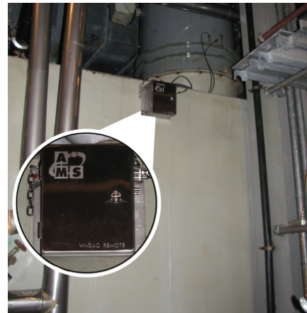
The WiDAQ System as installed in Nuclear Containment
